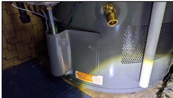
Safety pan and drain missing
